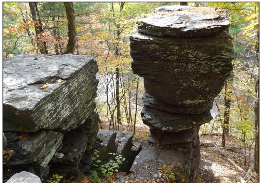
View to the southwest of Sentinel Rock from uphill. Tohickon Creek is in the background. The rocks dip gently 4 to 6 degrees to the northwest in this immediate area. The strike of the rocks is about 50 degrees northeast. Note the joint face on the rocks to the left.
